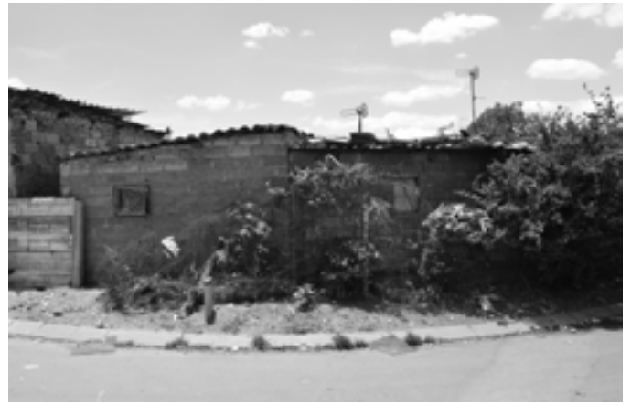
02. Boundary condition with houses built on and over property line
